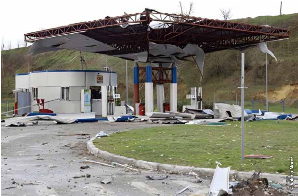
△ Destroyed gas station near Kyiv.
