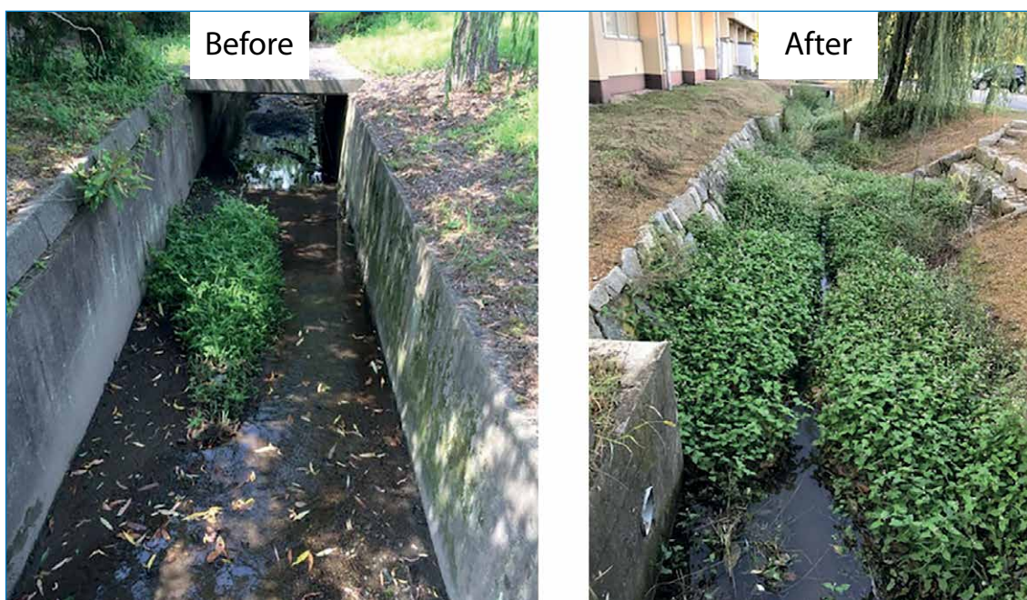
Figure 6: Before and after intervention: The image on the right shows a re-constructed drainage canal. (Image credit: © Mieko Kiyono)
